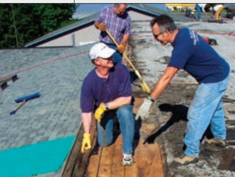
Members in Coeur d'Alene work to put a new pitched roof on the Lake City Junior Academy gym.
