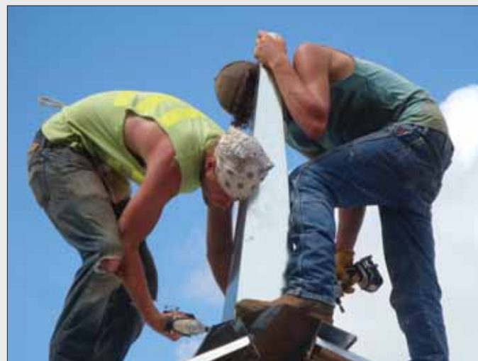
Adding a finishing touch, Colton Hayden and Logan Saterdal fasten the steeple to the newly completed Chilunguni Church in Malawi.
