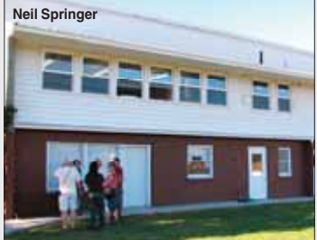
Enterprise School alumni and friends raised money to replace 30 windows in the classrooms and lunchroom, which had been installed in time for school tours at its first reunion.
