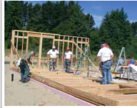
With Maranatha volunteers adding their talents to the project, the framework took shape quickly.
